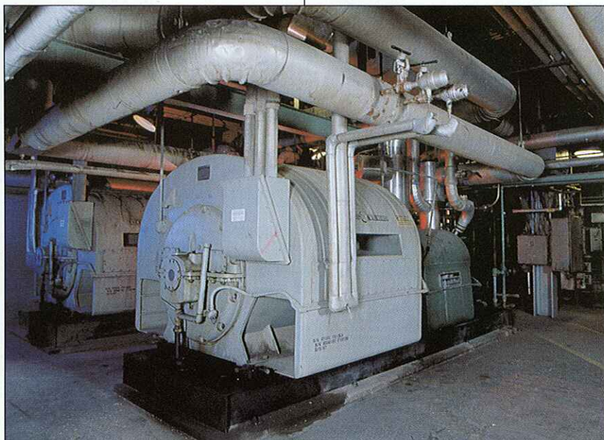
A variety of critical equipment, such as this boiler feedwater pump, is monitored to prevent motor failures and to ensure that the equipment starts without incident when a generating unit is brought into service.
