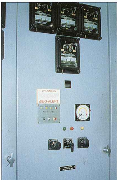
The insulation resistance tester display mounts in the switchgear panel. Readings are shown on a color-coded meter.
